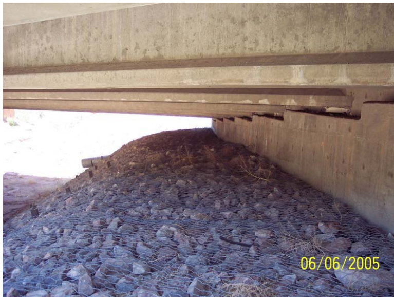
Figure 58 – Riprap used for Erosion Control (Lenke, 2006)
