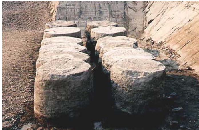
Figure 28 – Deep Soil Mixing (DSM) Operation and Extruded DSM Columns (Porbaha and Roblee, 2001)
