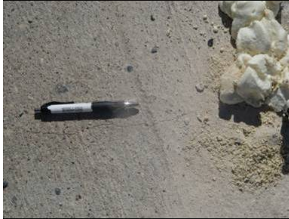
Figure 68 – Hairline Crack Observed on the Approach Slab during the Urethane Injection
