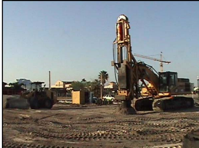
Figure B2 – Rapid Impact Compactor Used for Compacting 13 ft Thick Sand Layer for a Building Foundation ( www.terrasystemsonline.com )
