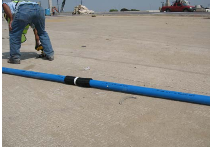
Figure 6.23. A Corrugated Pipe Was Placed on the Vertical Casing at Each Design Depth.
