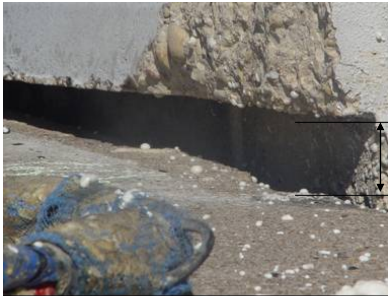
Figure 9.3. Settlement of the Approach Slab.
