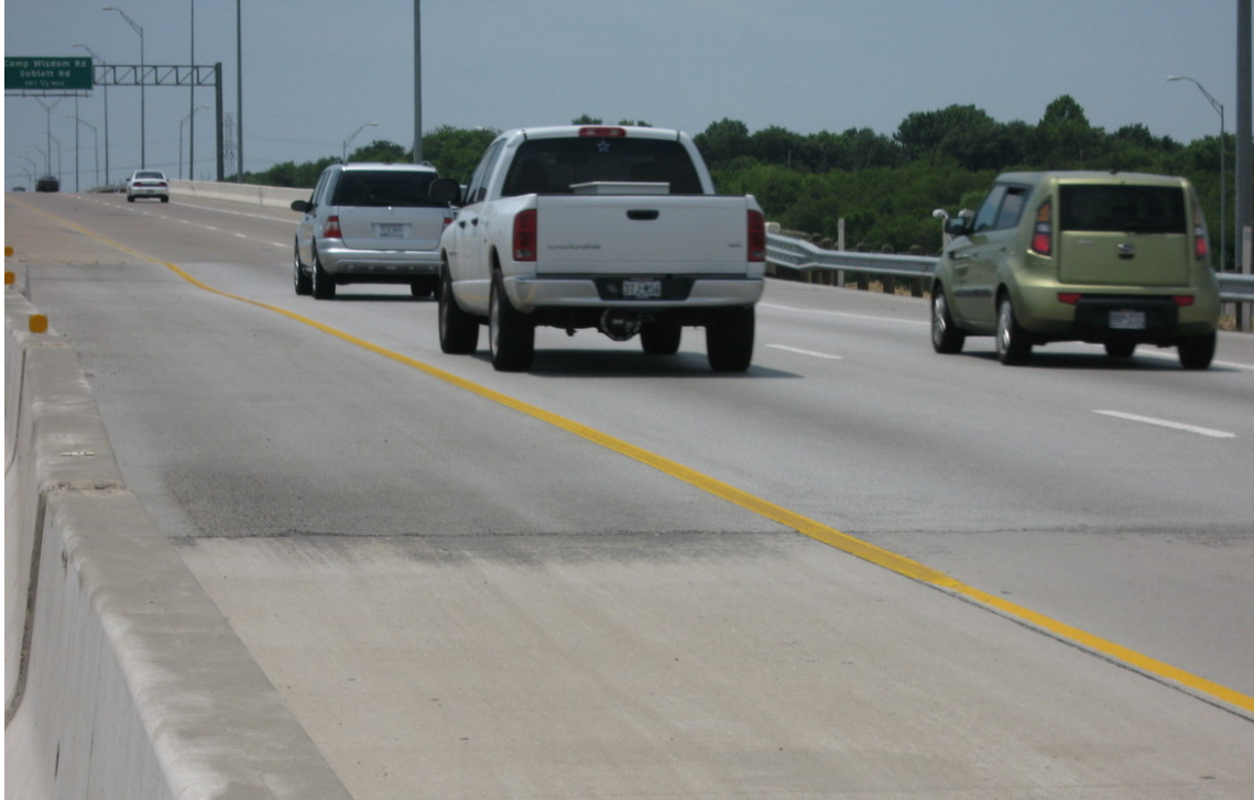
Figure 7.28. Bridge Approach in the Control Section Overlaid by Hot Mix Asphaltic Concrete to Mitigate the Bump.
