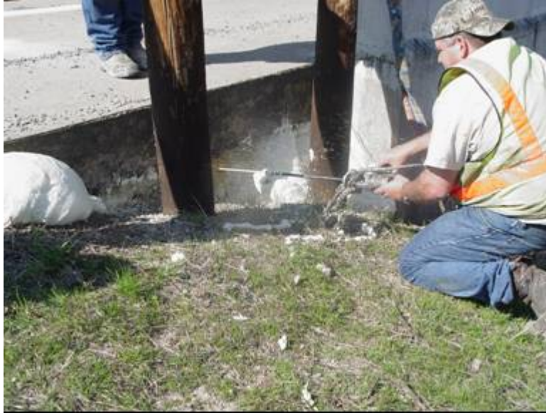
Figure 9.8. Sealing the Void from the Exterior Face to Protect Loss of the Injected Polyurethane.
