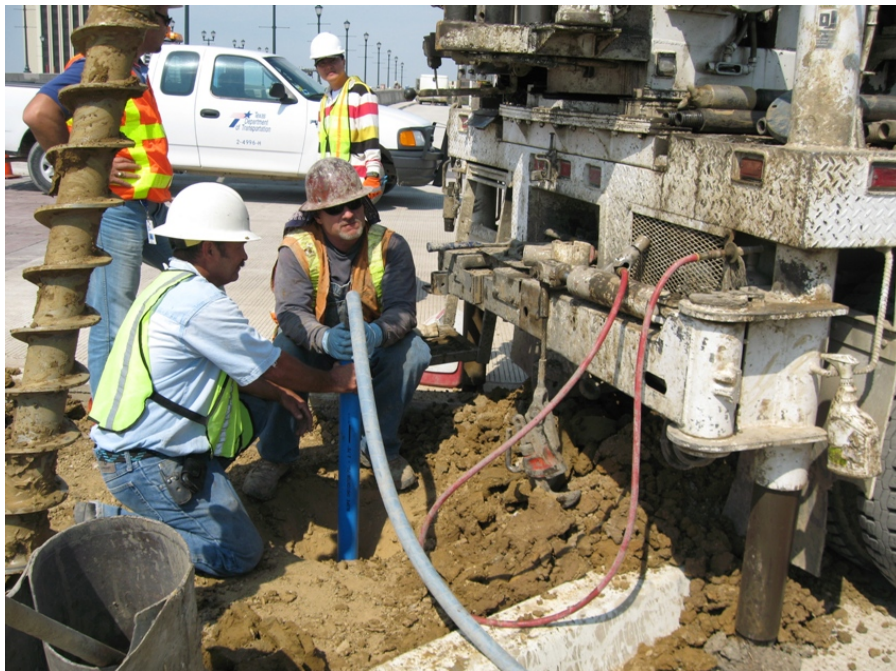
Figure 6.19. Water Was Filled into the Casing to Avoid Floating due to Buoyancy.
