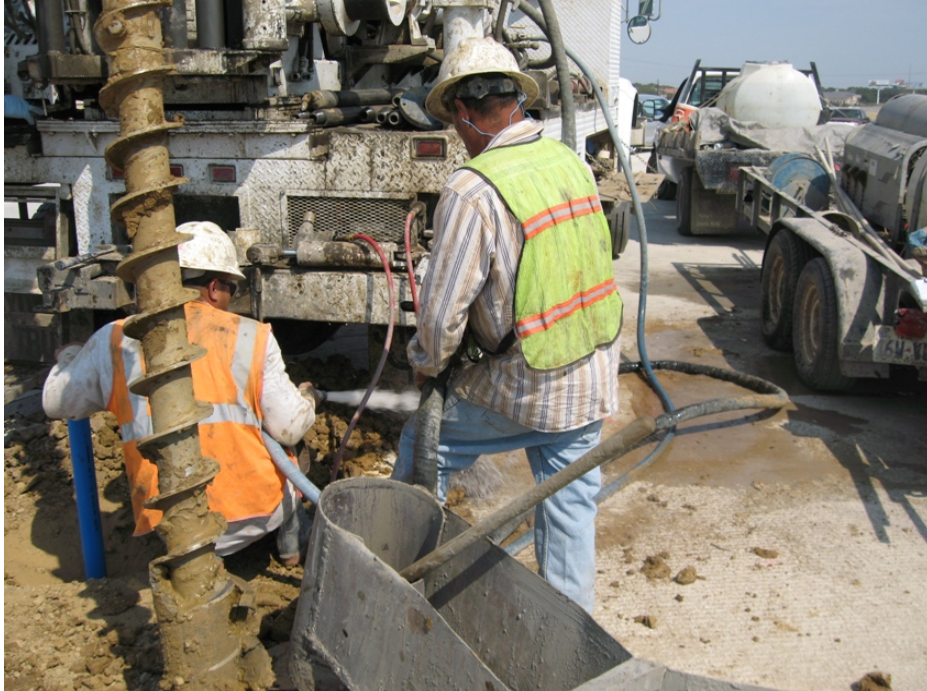
Figure 6.18. The Gap between the Casing and Borehole Wall Was Filled with Grout Mix.
