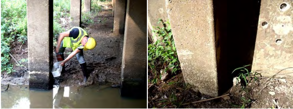
Figure B. 13. Overview of Bridge Deterioration (Bridge 1R).
