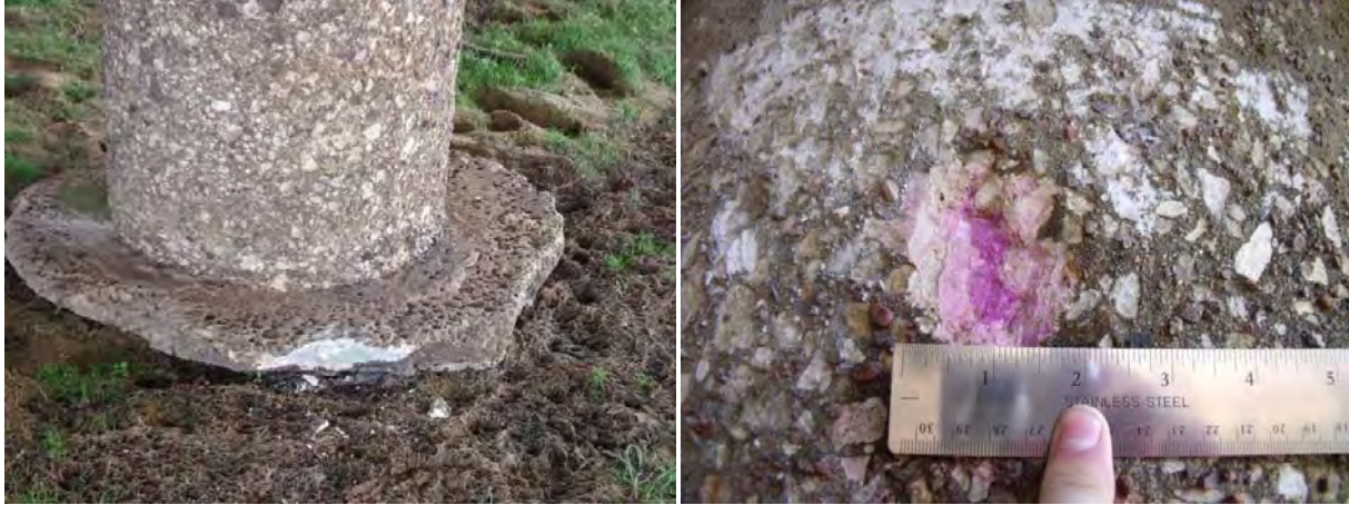
Figure B. 7. Overview of Bridge Deterioration (Bridge 7).
