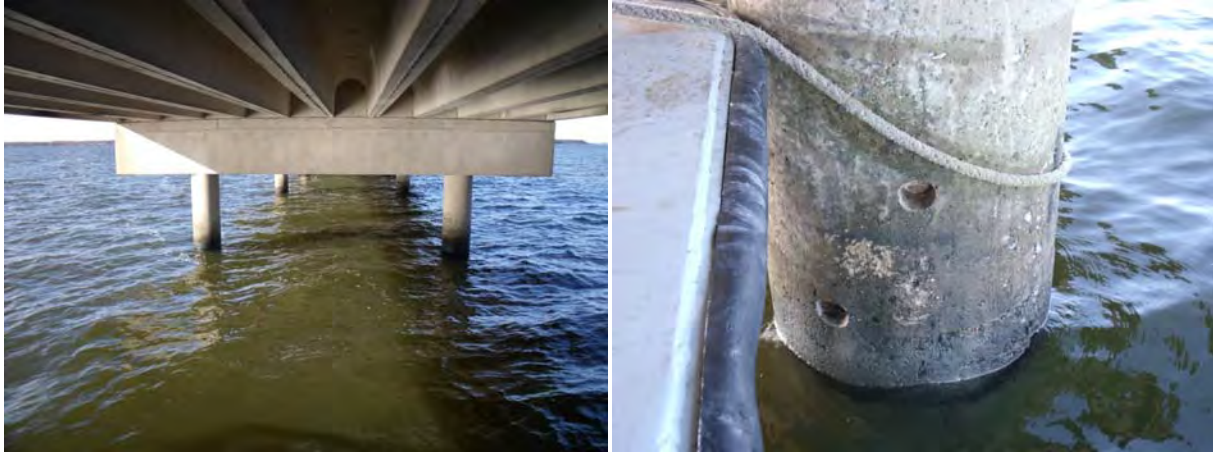
Figure B. 3. Overview of Bridge Deterioration (Bridge 3).
