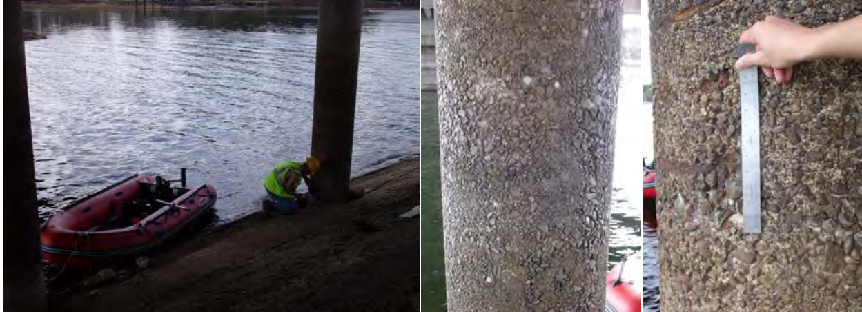
Figure B. 6. Overview of Bridge Deterioration (Bridge 6).
