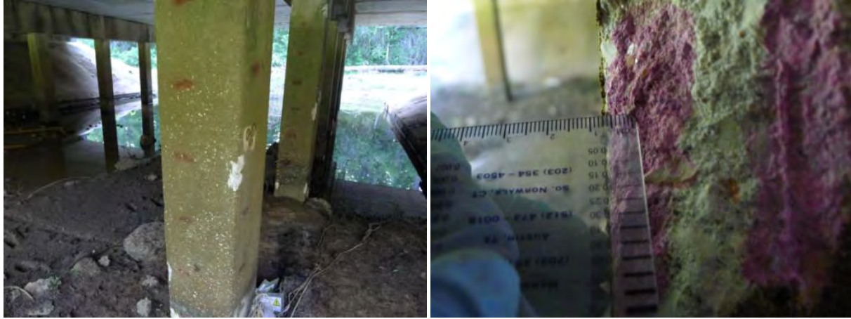
Figure B. 10. Overview of Bridge Deterioration (Bridge 10).
