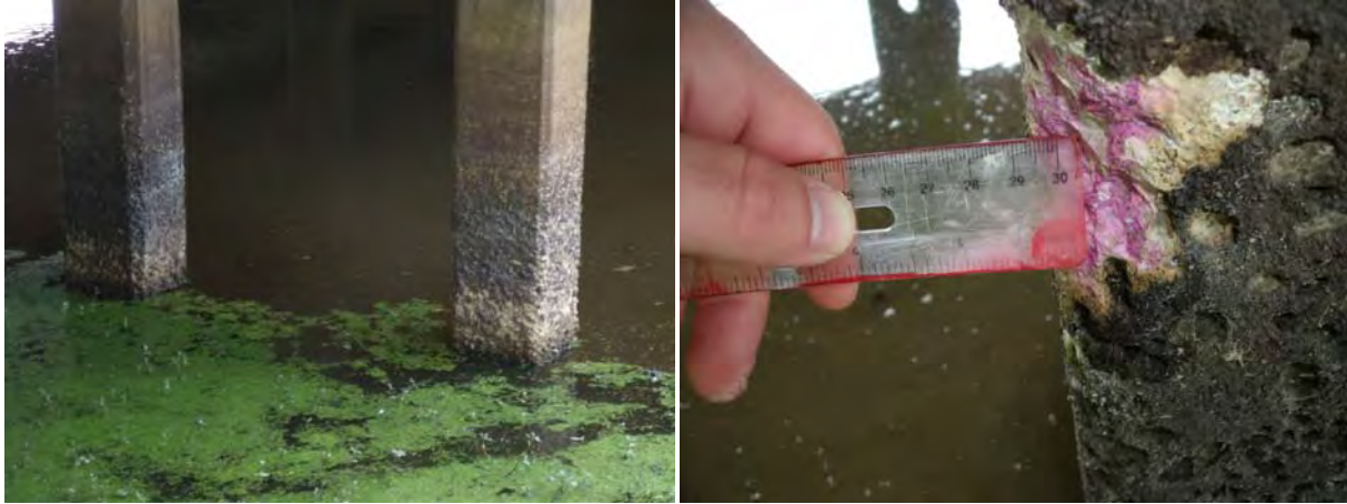
Figure B. 9. Overview of Bridge Deterioration (Bridge 9).
