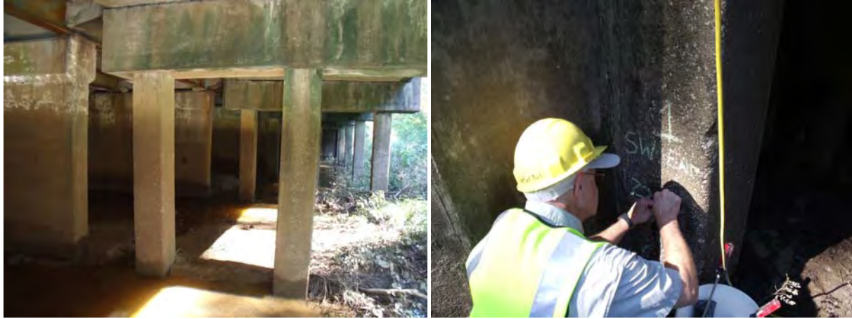
Figure B. 1. Overview of Bridge Deterioration (Bridge 1).
