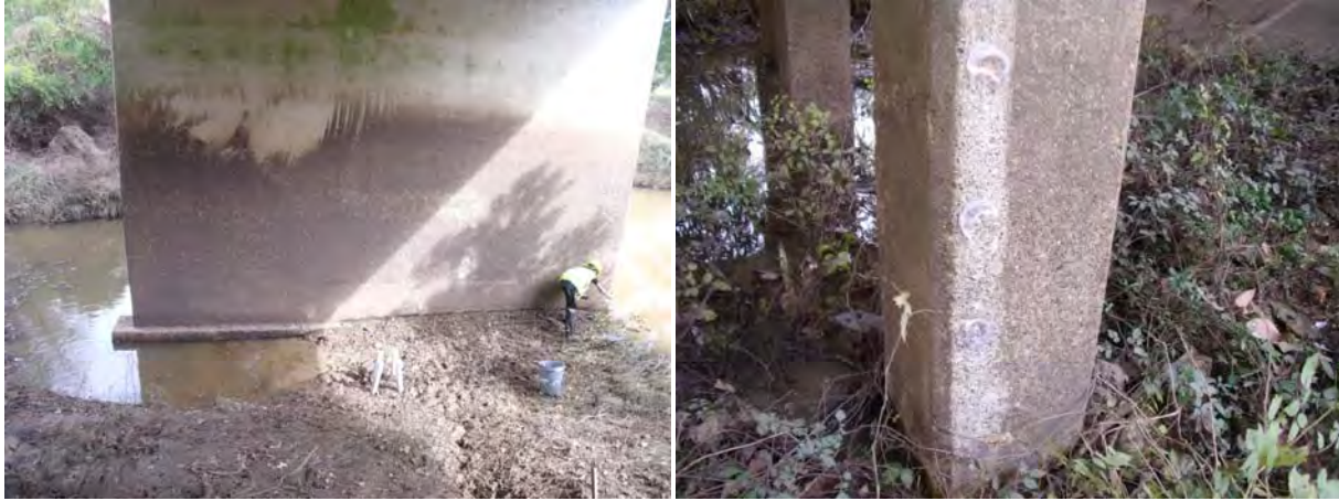
Figure B. 2. Overview of Bridge Deterioration (Bridge 2)
