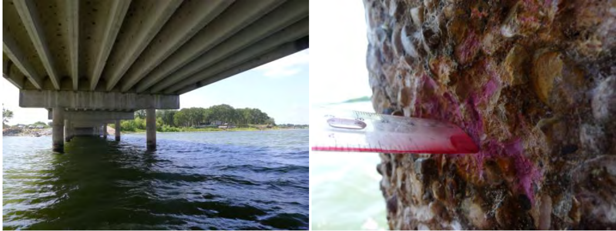
Figure B. 12. Overview of Bridge Deterioration (Bridge 12).
