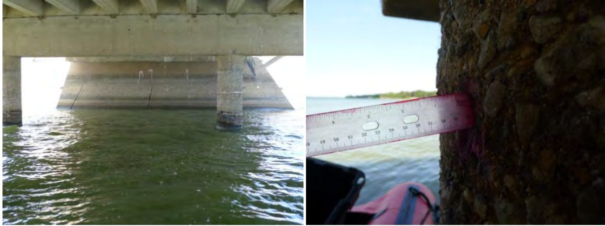
Figure B. 11. Overview of Bridge Deterioration (Bridge 11).
