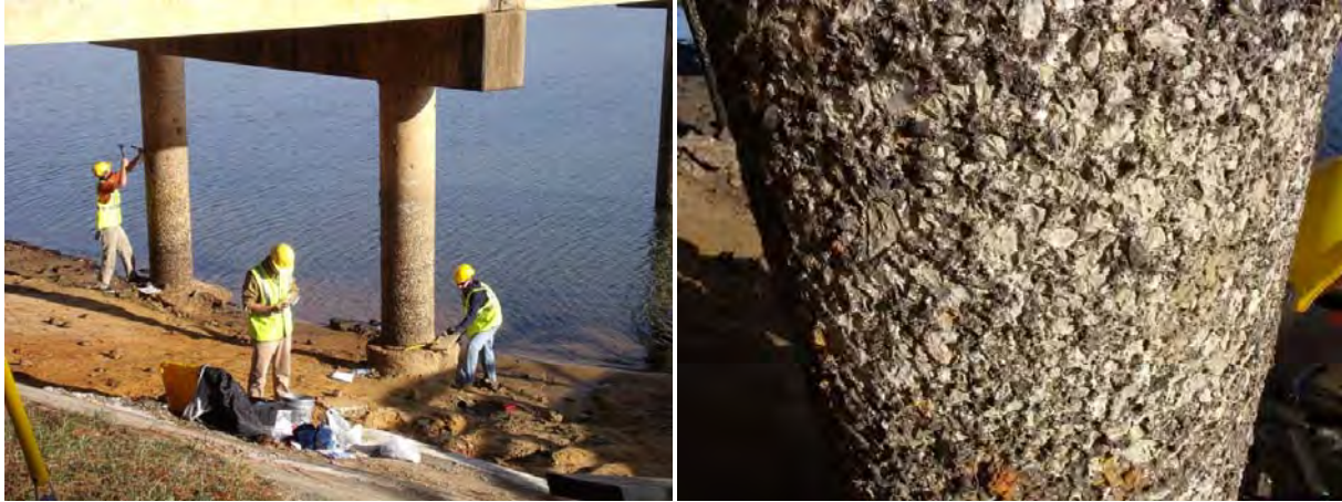
Figure B. 5. Overview of Bridge Deterioration (Bridge 5).
