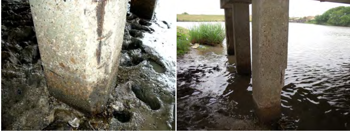
Figure B. 4. Overview of Bridge Deterioration (Bridge 4).
