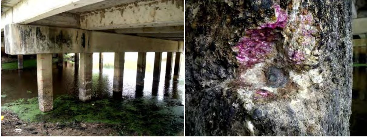
Figure B. 8. Overview of Bridge Deterioration (Bridge 8).
