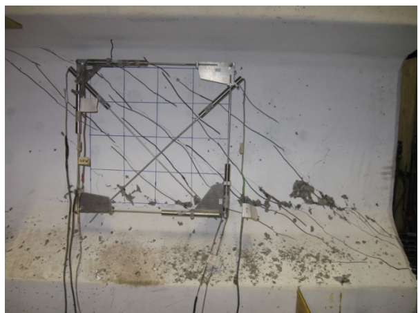
(f) Shear failure at 912.78 kips
