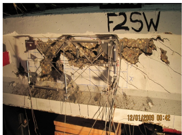
(f) Shear failure at 185.35 kips
