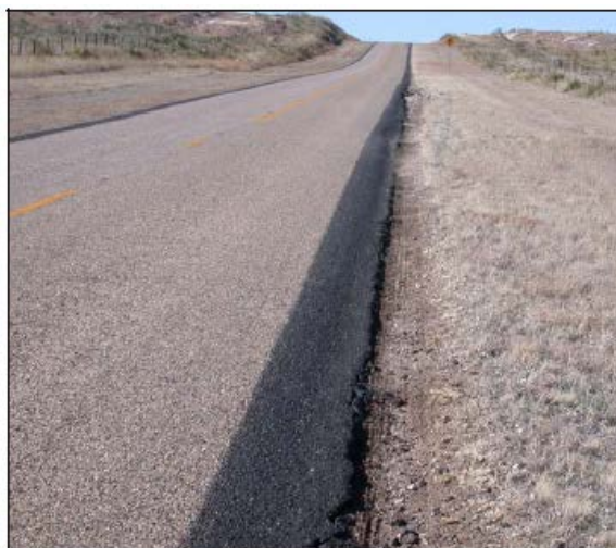
Figure 2.8. Pavement edge drop-off.
