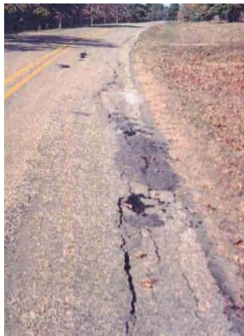
Figure 2.1. Longitudinal cracking and failure (Sebesta 2005).
