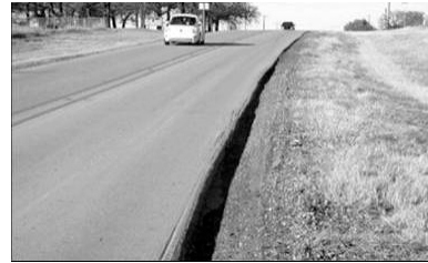
(b) Edge drop-off due to erosion
