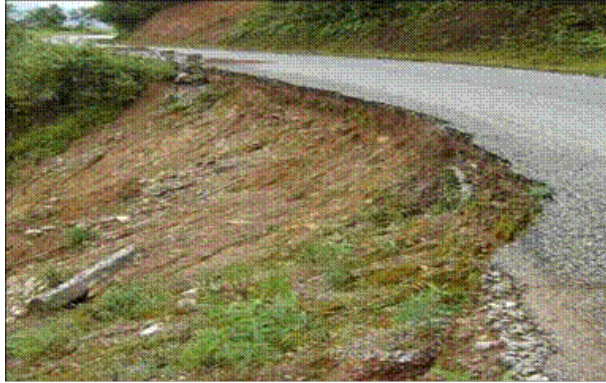
Figure 2.4. Edge Failure due to Slope Instability (Hearn et al. 2008).
