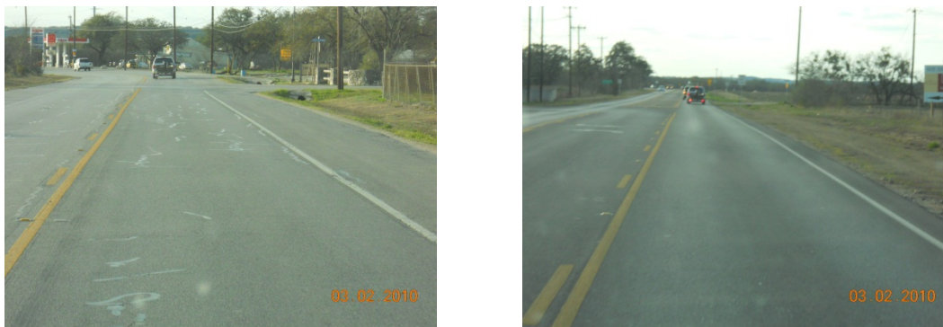
Figure 4.11. Surface Condition Showing Rutting and Cracking in the Wheel Path at the Control (left) and Distress-Free at the Reconstructed (right) Sections.
