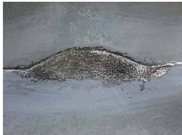
(d) Repair weld after application of UIT to both the face of the weld and toe
