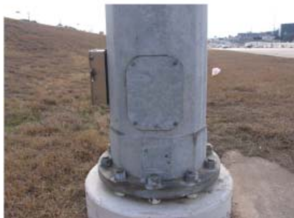
Figure 2. Winch System Access Hatch (Stam, 2009).
