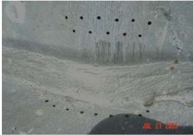
(a) Visual appearance of apex with UT indication of lack of weld fusion (no visible fracture)
