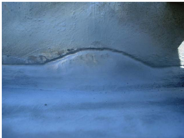
(c) Repair weld made to improve fatigue life. The profile meets the requirements of AWS D1.1. Toe dressing has been performed at the weld toe
