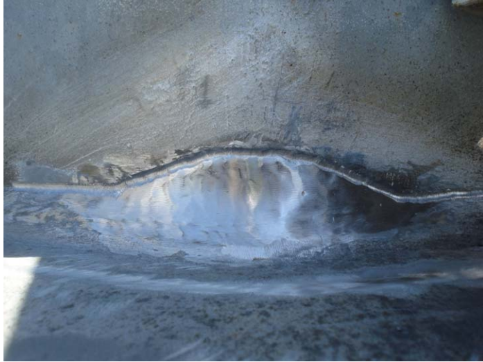
(a) Weld repair with toe dressing (prior to UIT) (courtesy Lamb-Star Engineering LP)
