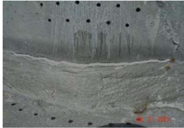
(b) After removal of galvanization by grinding at weld toe (no visible fracture)
