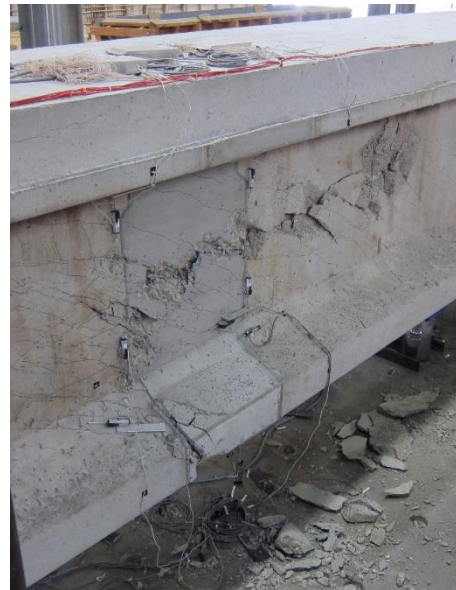
Figure 1. Phase II Spliced Girder Specimen after Failure.
