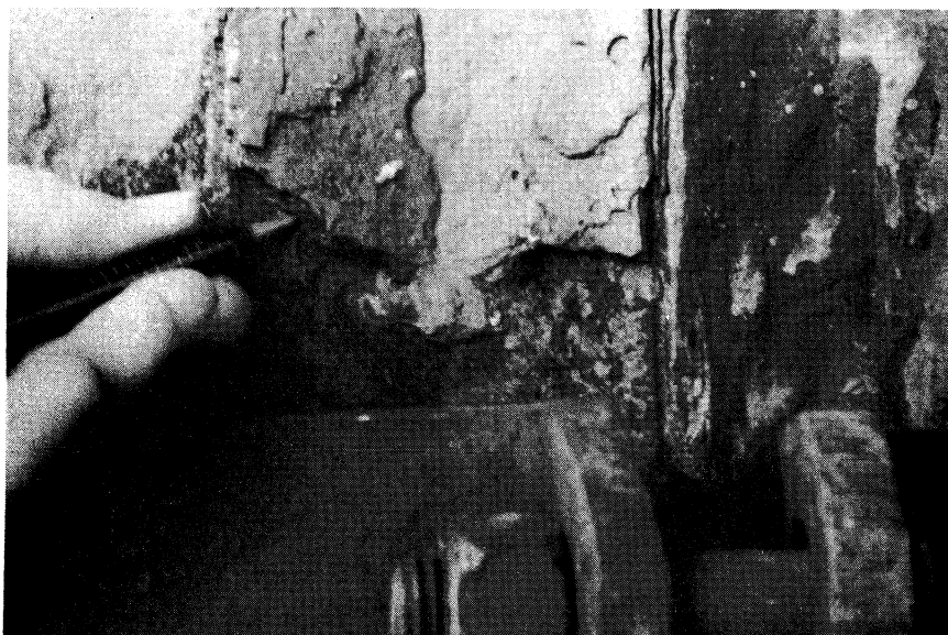
Figure 11. Bay side view of corroded piling at a point 6' above the water line showing rust fracture line at flute intersections.
