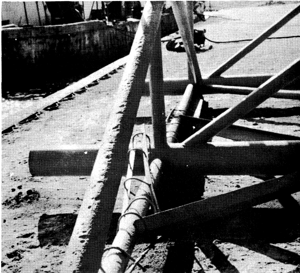
Figure 14. Structure removed from salt water showing excessive corrosion of member in foreground; this member was located at the mud-water interface.
