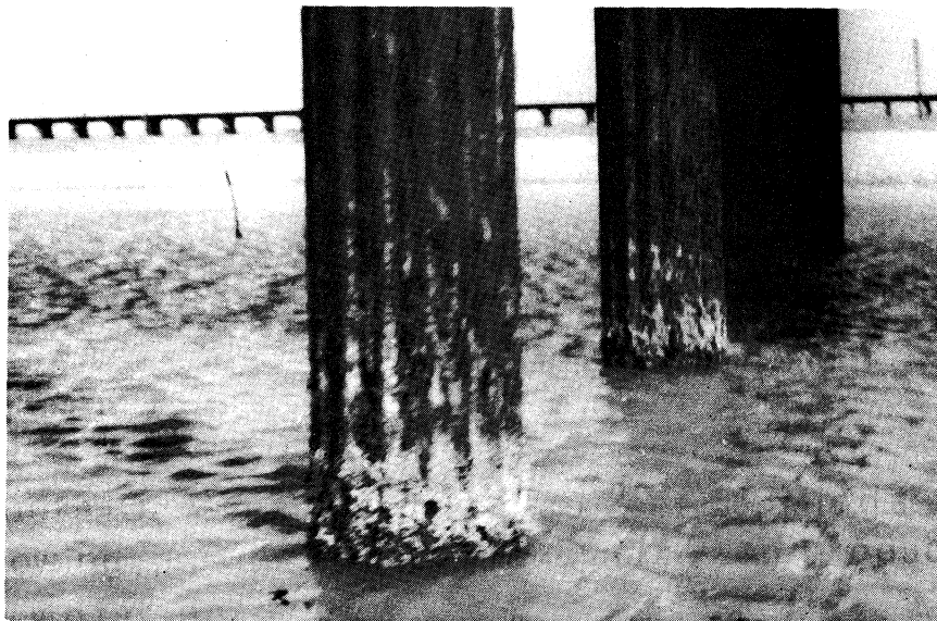
Figure 10. General view of corroded pilings showing marine growth and corrosion product at water line.
