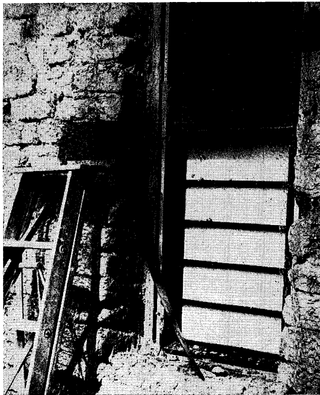
Figure 20. The nailer block in Figure 19 is shown in place (under the building paper) in this residence under construction in Albuquerque, N. M. (Koeber).
