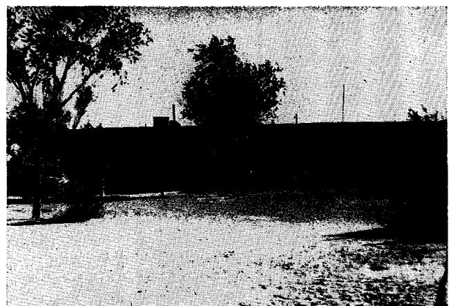
Figure 8. Straw from adobe blocks in this 100-year-old community building at Ysleta, Texas, showed no signs of rot or deterioration.
