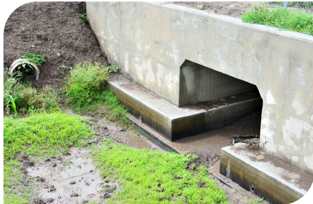
Figure 3.7. Small/medium animal underpass box culvert (ca. 1.5 x 1.5 m, w x h) for ocelots along FM 106 at Ted Hunt Road, Texas (Kelley 2018)
