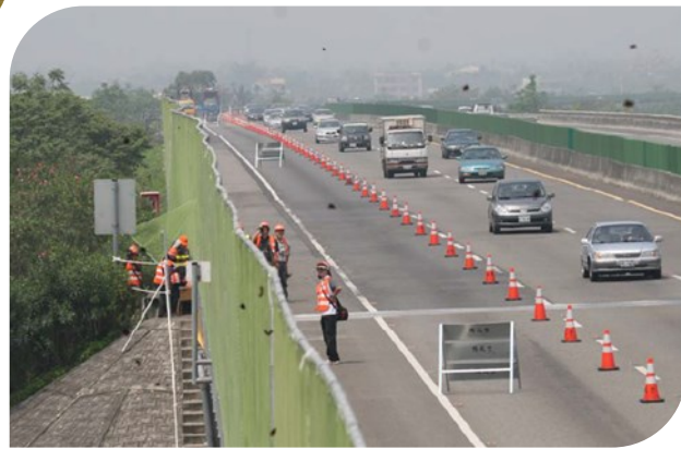
Figure 4.9. Outer lane closure on Chingshue Brook Viaduct of National Freeway 3 in Taiwan during purple crow butterfly migration (TAFNB 2008)
