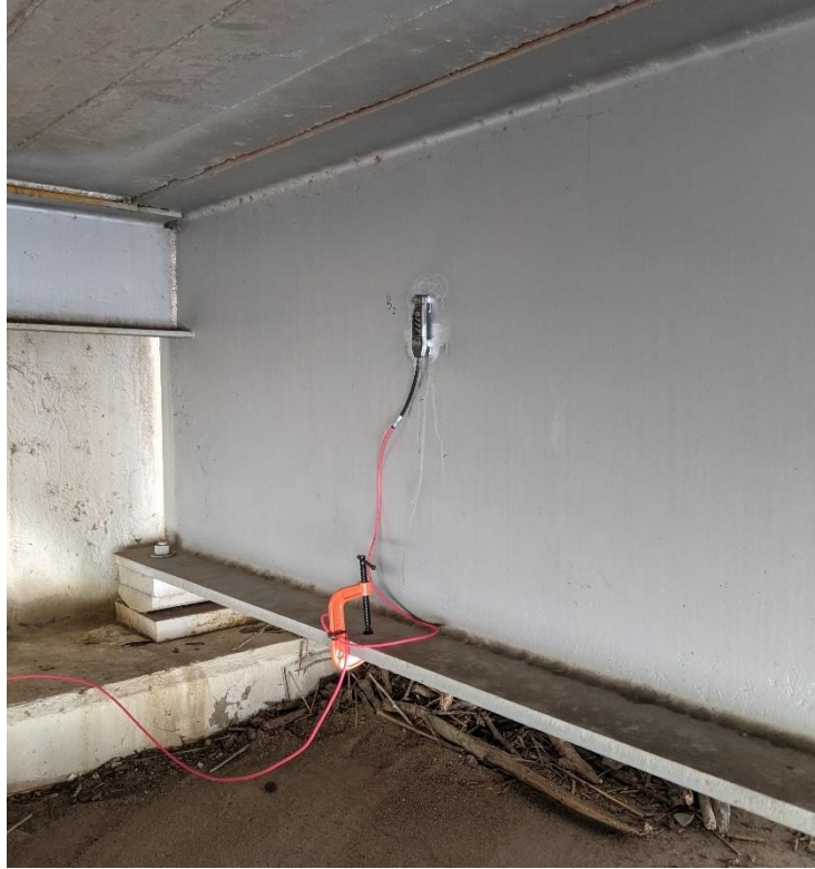
Figure 5.32. Vertical Strain Gauge at North End (Bridge #3).
