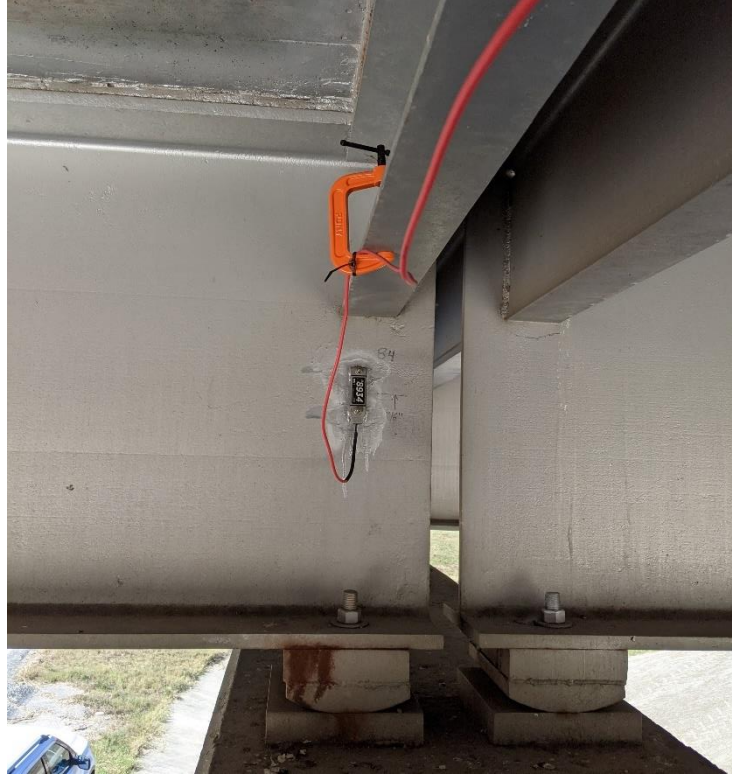
Figure 5.30. Vertical Strain Gauge at Second Span (Bridge #3).
