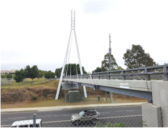
(a) Instrumented Bridge
